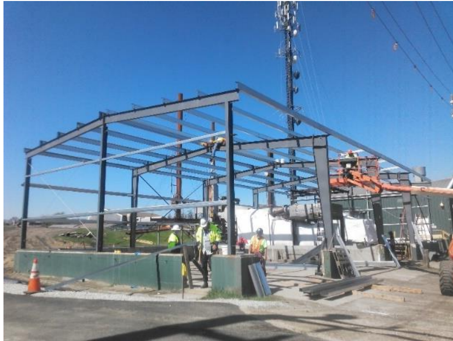
Block Island Power Plant
